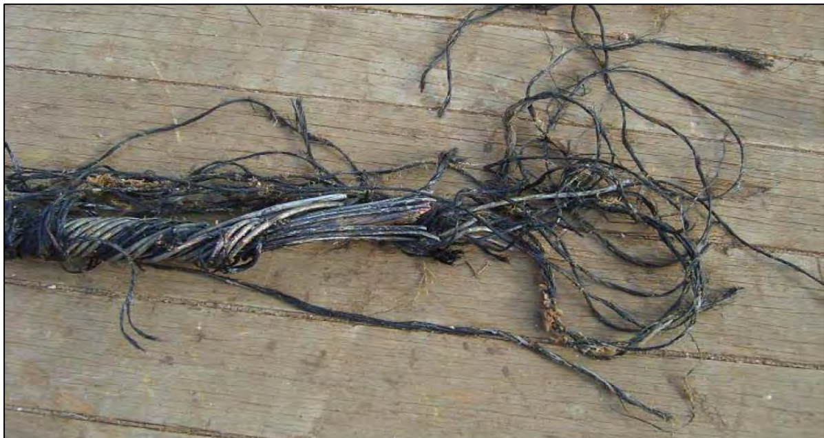
Figure 48 Cable Fault Caused by Fishing Gear (UK-NL14, Repair 4, May 2011)
